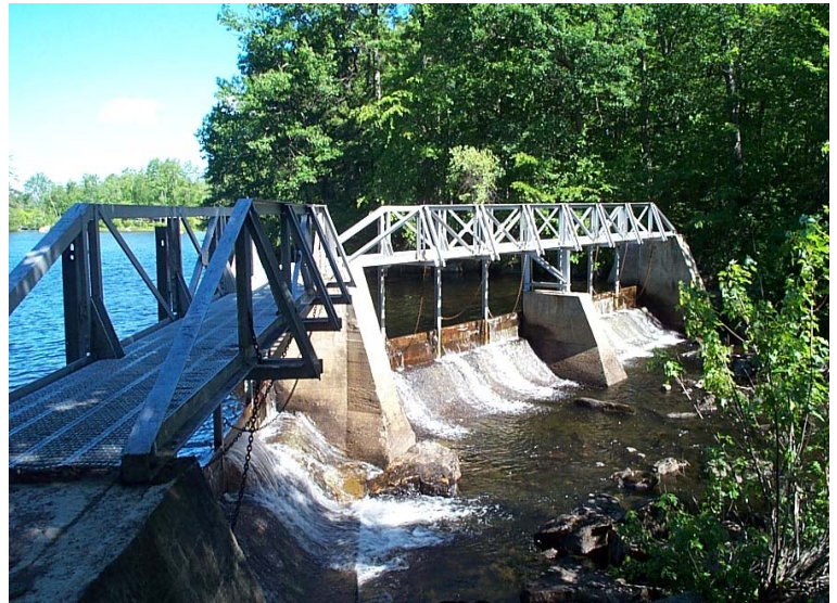
One of two sections of the Ossipee River dam, which has controlled the height of the lake since being constructed in 1911. Alliance Photo
